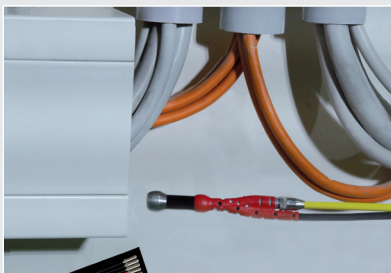
Shafts and underfloor ducting
